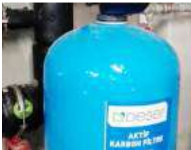
Automated valve filtration systems with FRP tanks
